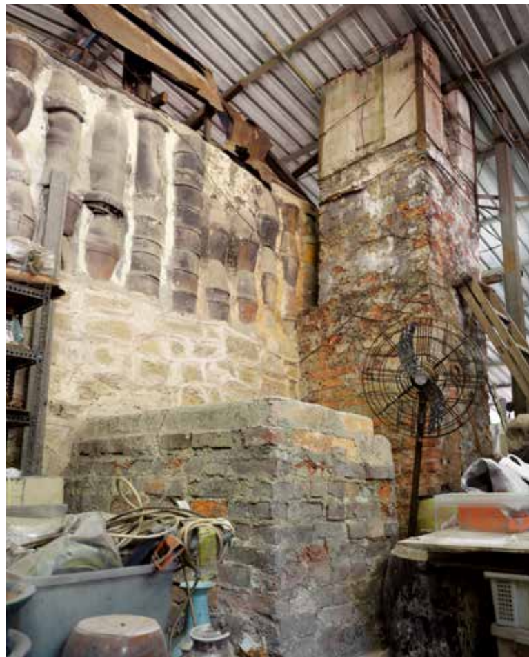
煙囪旁邊的「加力燃燒室」，相信是經改建的結構，有助保留熱力，減短燒窯時間。 The afterburner is likely a later edition and helped speed up firings.
